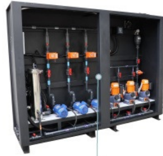
Brine Proportioning Unit
